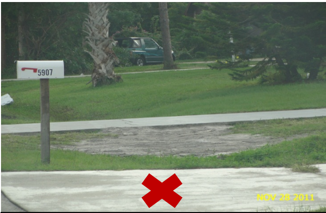
Swale filled in with dirt
