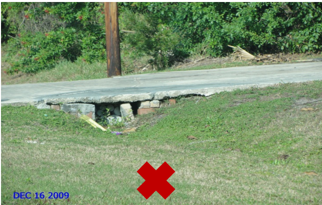
Culvert failed and swale is blocked by debris supporting the driveway
