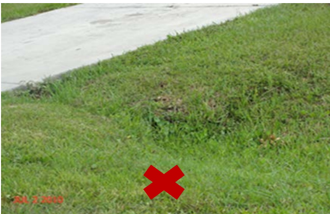
Driveway culvert blocked with grass
